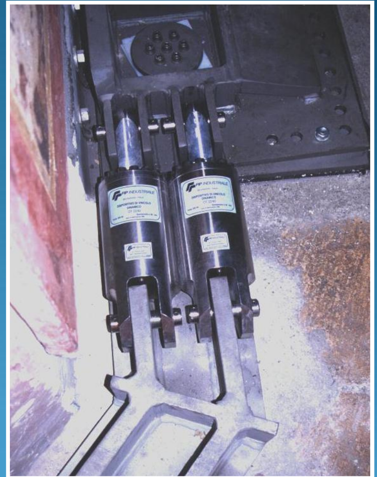
Shock transmitters installed between nave and transept
