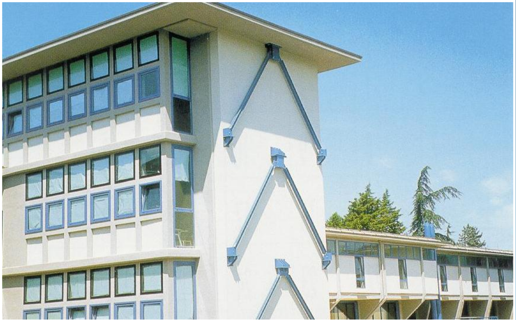
Dissipative braces in one school in Fabriano
