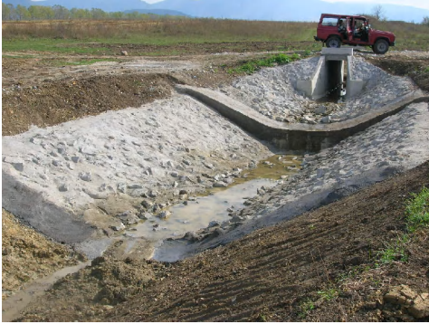
Photo 15 – Pipe DN1200 (of caissons) and drop of concrete and rough stone on drainage channel CS403 (2008)
