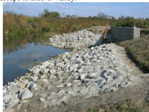
Photo 24 – Lisava Valley Under-crossing the dike with metallic damper on channel CCS43 (2008)
