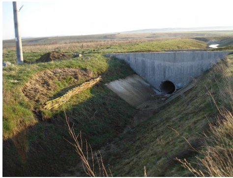
Photo 5 – Culvert pipe DN1000 on CCS43 Consolidation of slopes with fences of wattle (2010)
