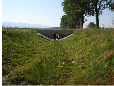
Photo 16 – Pipe DN1200 on drainage channel CP41 (2010)
