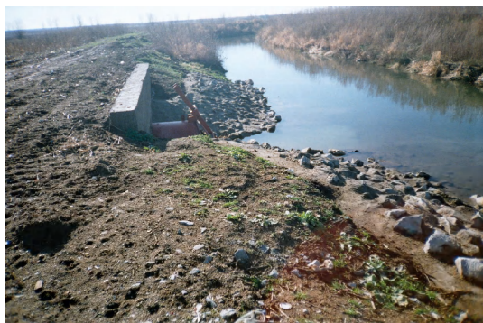
Photo 23 – Lisava Valley Under-crossing the dike with metallic damper on channel CCS42 (2008)
