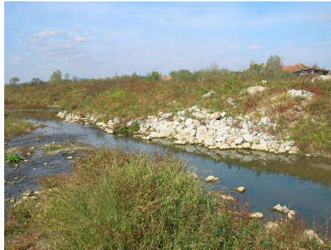
Photo 20 – Lisava Valley Consolidation with rough stone at the junction with cu Oravita Valley (2010) Oravita Valley and three Lisava Valley;
