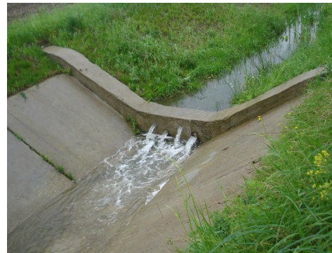
Photo 18 – Threshold drop of concrete on drainage channel CS403 (2010)
