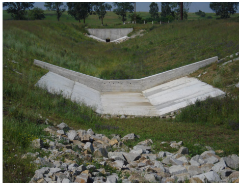
Photo 17 – Threshold drops, pipe DN1000 and consolidation at the junction with Lisava Valley of drainage channel CP41 (2010)
