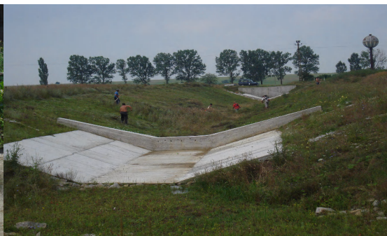
Photo 4 -Main drainage channel CP41 threshold drop of concrete, works for the destruction of aquatic vegetation and grassy (2010)
