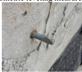
Figure 8. Survey marker fixed to the monitored object
