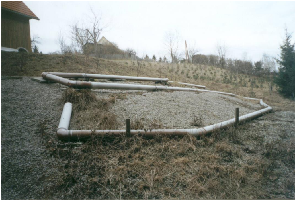
Figure 3.2. Plant-based water filter, distribution pipe and filter bed substrates
