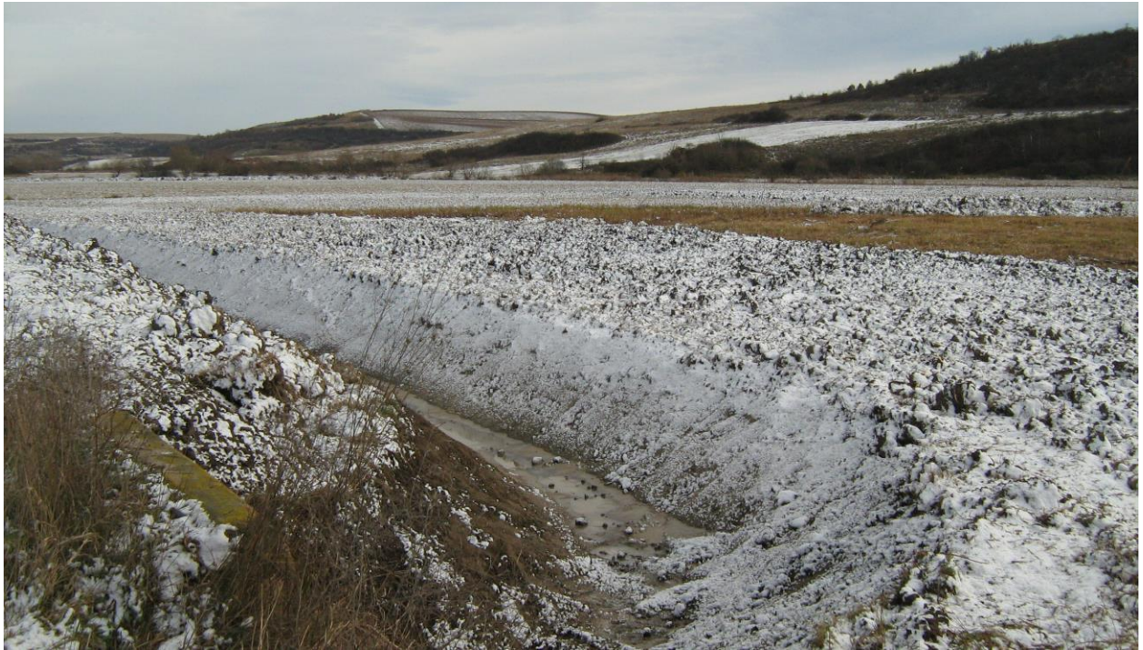
Figure 2. Operational exhaust channel
