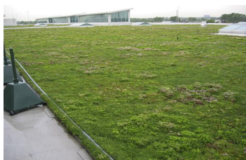
Fig. 18 Portion of extensive green roof on an assembly plant at Ford Motor Company in Dearborn, Michigan. Plant material consists of 13 species and cultivars of Sedum (Photo by Brad Rowe).
