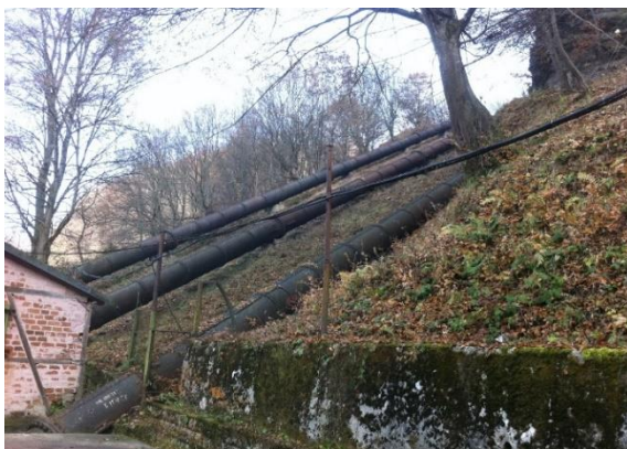
Figure 8. The three penstock metal pipes
