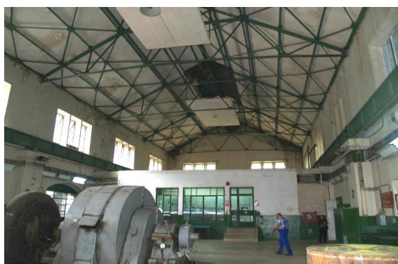
Figure 5. Machinery room at Grebla HPS, previously the rehabilitation process
