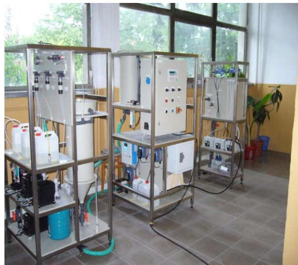
Figure 3. Water purification unit by microfiltration, UPT, Department of Hydrotechnical Engineering
