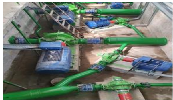
Figure 8. Interior view SPP10 after installation of new pumps and related fittings (Photo Cioclov)
