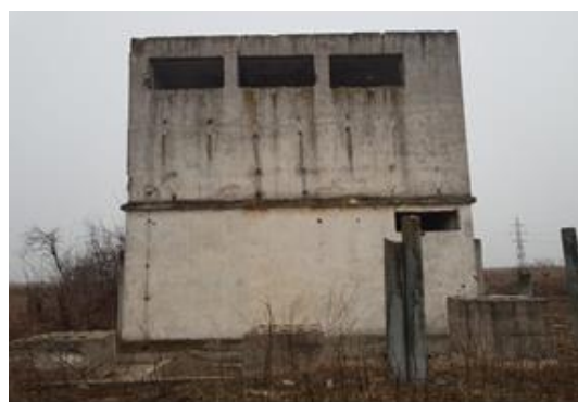
Figure 2. Overview of the SPP10 side facade with missing impact demand (Photo Cioclov)
