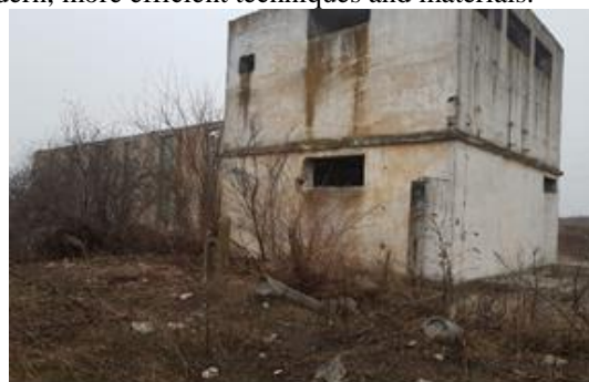
Figure 1. Overview of degraded SPP10 (Photo Cioclov)
